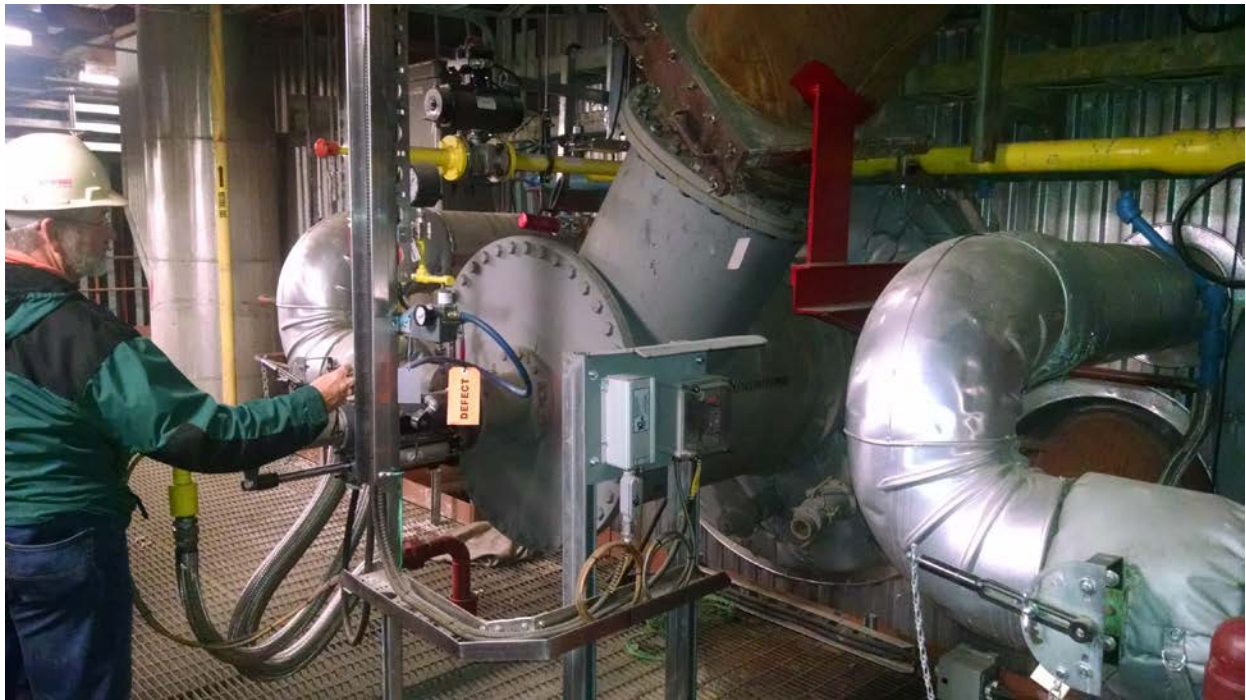
Pulverized Pellet Fuel Burner in the Atikokan Power Plant
